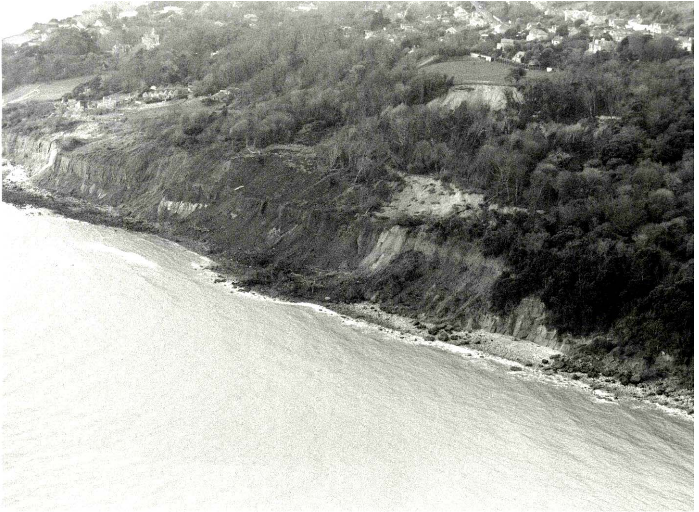
Figure IW29.2.1 ‘The Landslip’, Bonchurch, encroaching towards Bonchurch village and the road to Shanklin.
