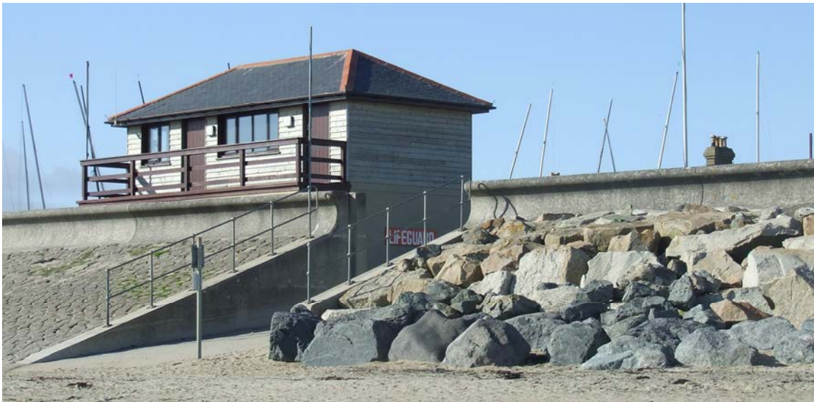
Above: Defences at Marazion – a concrete wave return seawall is fronted by both rock and concrete sloped revetments
